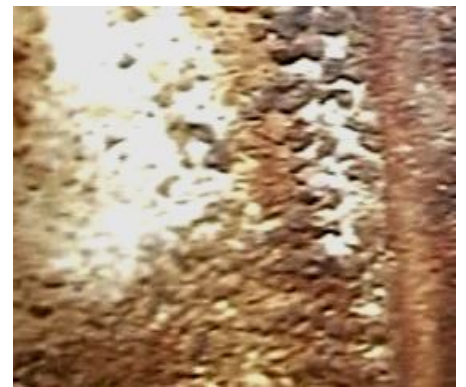
Operator Observation: Surface Damage
